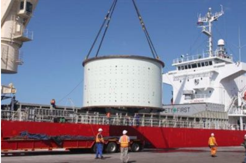
Figure1. Loading SAG mill shell for transport to Australia (which has subsequently arrived in Australia and is ready for transport to site).
