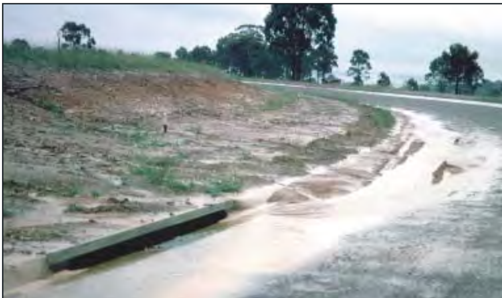
Figure 6.2 Sediment resulting from unsatisfactory rehabilitation following roadworks
