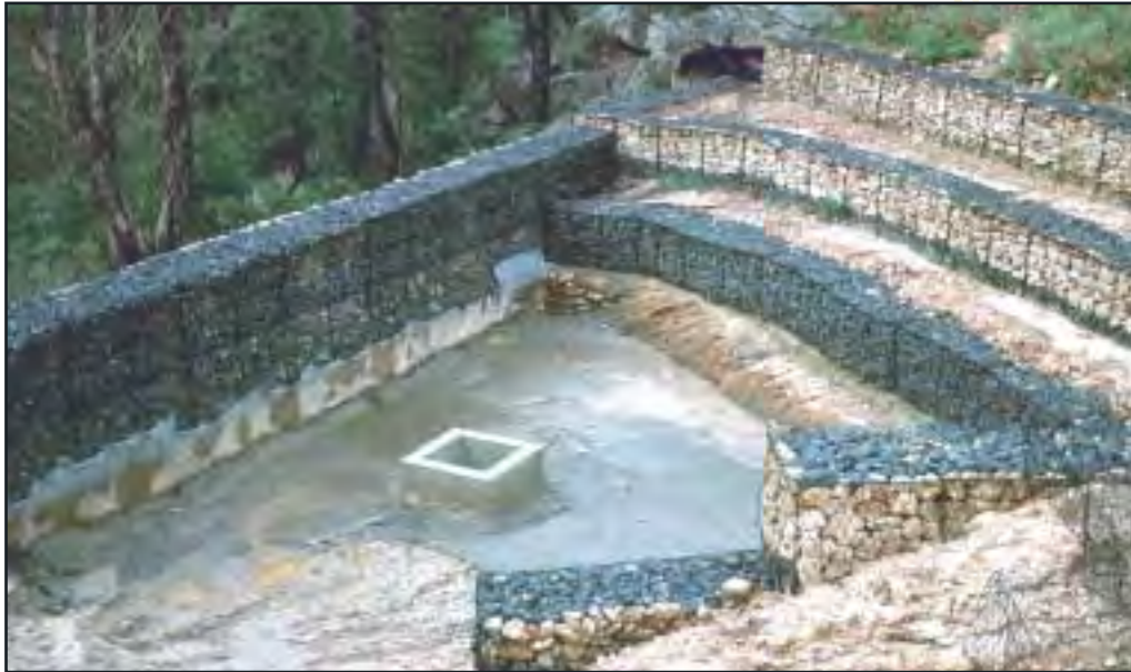
Figure 6.7 A sediment retention basin constructed on Type C soils with gabion baskets in very steep country. The structure has recently been converted to a constructed wetland.
