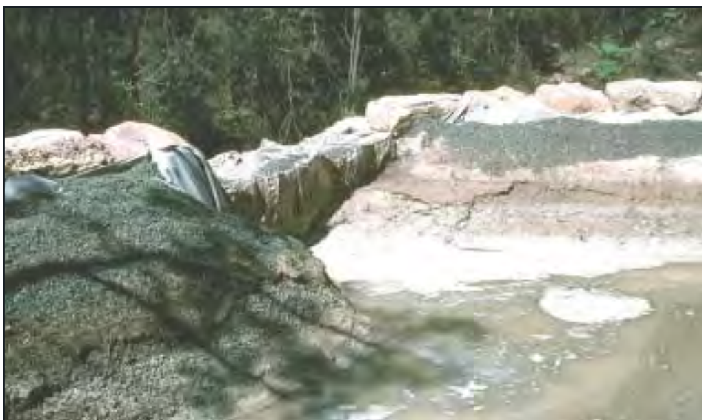
Figure 6.8 A sediment retention basin constructed on Type C soils from local sandstone gibbers
