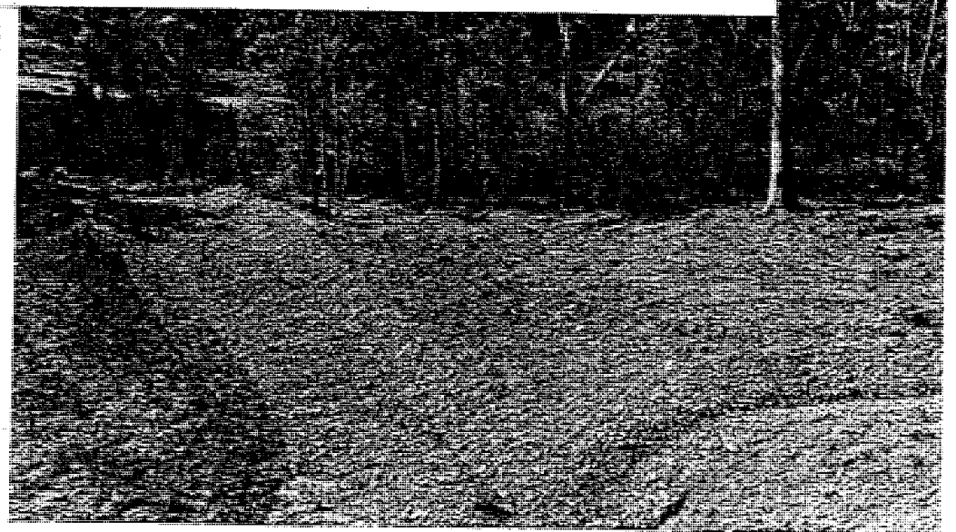
Temporary and permanent channel linings stabilise drainage channels against erosion.
