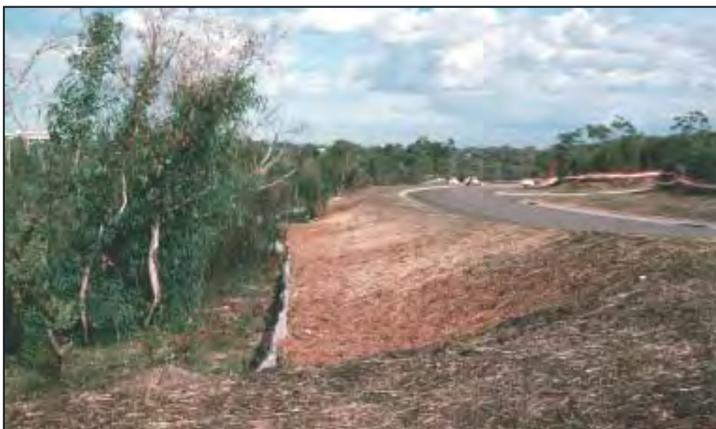
Figure 7.2 Primary revegetation of an earth batter with straw mulching (Section 7.4.1). Notice the sediment fence and barrier mesh to minimise soil erosion and sediment pollution
