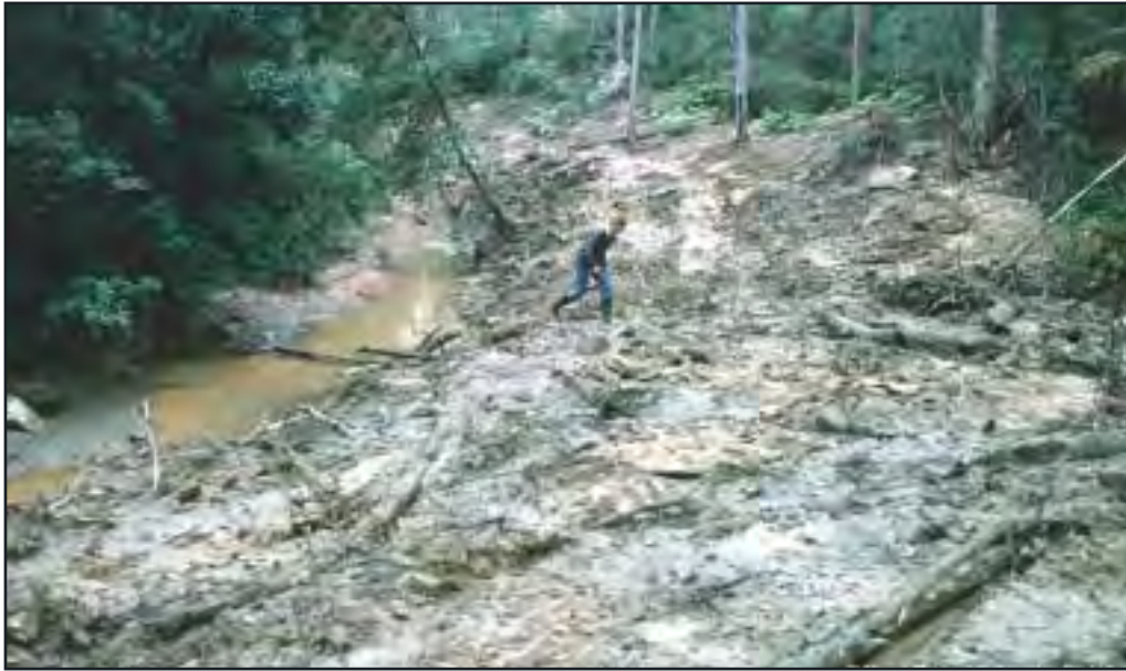
Figure 7.4 Lack of site stabilisation of a drainage line following installation of services
