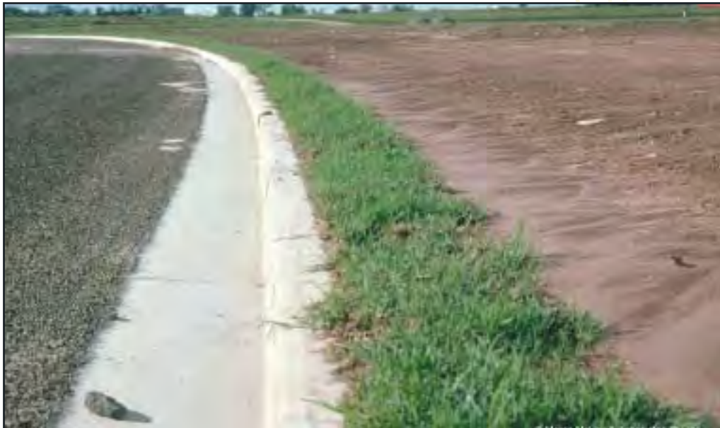
Figure 6.12 A kerbside turf strip showing sediment stored in the area above the filter.
