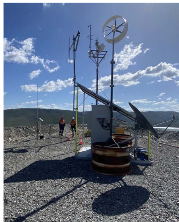
Solar and wind powered weather station at Mt Rawdon
