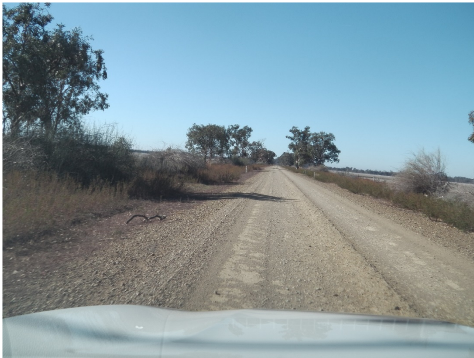
Photograph A.40 Bogies Island Road westbound, gravel surface with excellent sight distance
