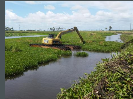
Burdekin waterway improvement at Kalamia Creek to reinstate an open body of wetlands, restore fauna diversity and improve farm productivity
