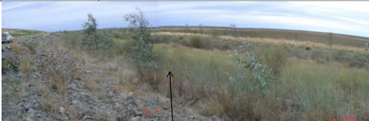
Temporary Isolation Bund - establishment of natural vegetation providing protection and stabilisation of the outer bund wall from the waters of Lake Cowal (when the lake bed was inundated).
