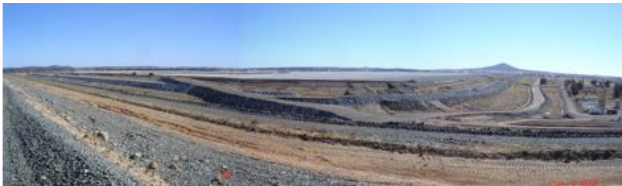
NTSF new lift construction during 2015/16 with TSF walls modified to meet the Tailings Management Standard for earthquake stability.
