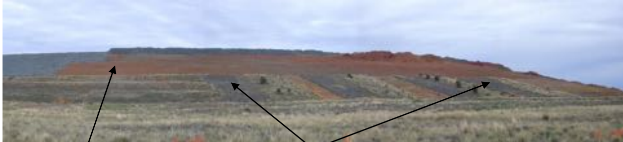
SWRE establishment of vegetative growth on the trial plots April 2015 and shaping topsoiling of the upper batters readied for revegetation of the upper slopes that have reached the finished RL. .
