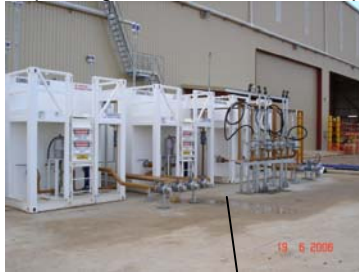
Plate 2: Oil/Grease storage and dispensing units for Fleet Workshop
