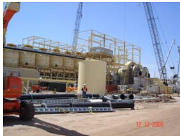
Plate 4: Flotation tanks – process plant
