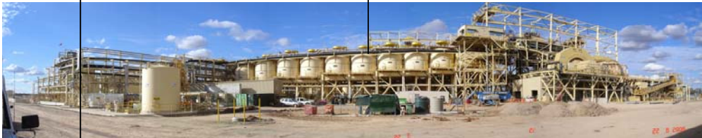
CGP ore processing plant - May 2008.
