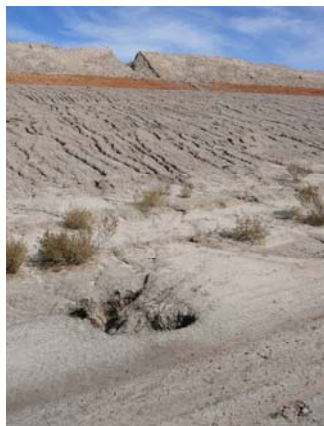
Plate 2: Erosion on the lake protection bund from recent rainfall runoff.
