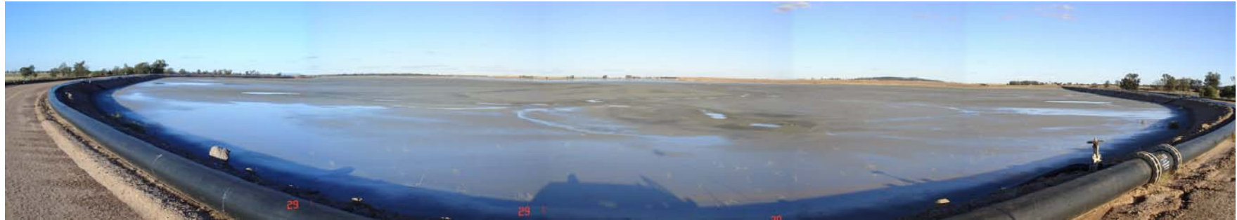
Northern Tailings Storage Facility (looking southeast from the north west corner of the NTSF) May 2008
