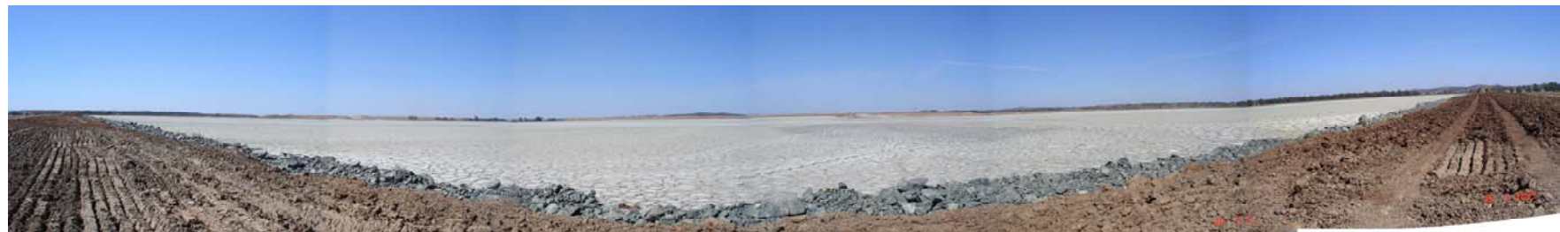
Northern Tailing Storage Facility during construction of the next lift (looking southeast April 2009).
