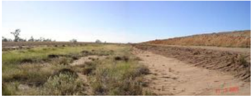
Plate 3: Road maintenance repaired erosive deterioration of the access track on the southern side of the Lake Protection bund and revegetation between the 'temporary' bund and the access track is well established stabilising the reactive soils.
