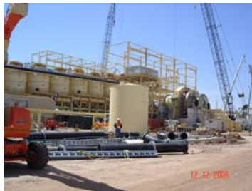
Plate 4: Flotation tanks – process plant
