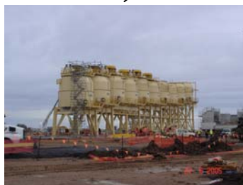
Plate 4: Flotation tanks – process plant
