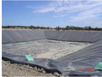
Plate 2: Contained Water Storage D6 – HDPE lined.
