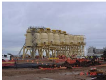
Plate 4: Flotation tanks – process plant
