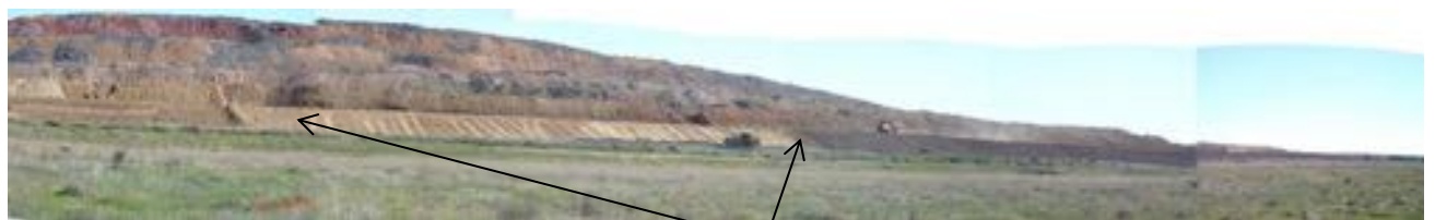
Rehabilitation works adjacent to Pond D1 using the rock-topsoil method for revegetation of the lower batters.
