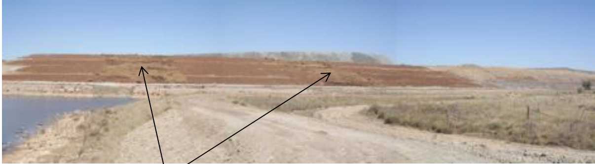
Plate 10: Rehabilitation trial on the perimeter waste emplacement with contouring and using straw bale substrate to control erosion and retain soil for vegetation establishment
