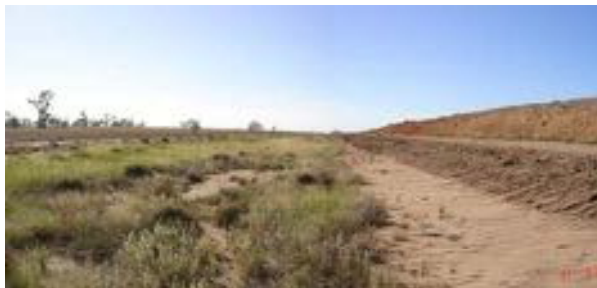
Erosion along the side of the access around the lake bund wall March 2009
