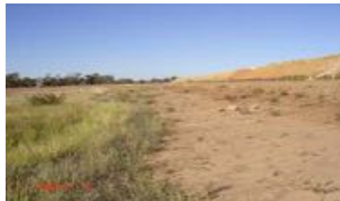
Erosion along the side of the access track around the lake bund wall repaired April 2010
