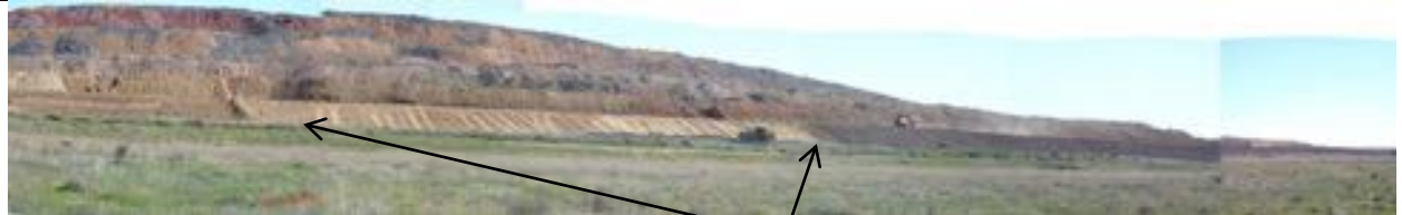
Rehabilitation works adjacent to Pond D1 using rock-topsoil method for revegetation of the lower batters.
