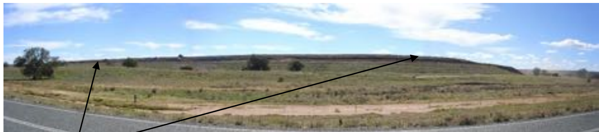
STSF outer batter being strengthened with rock emplacement to meet the Barrick policy of tailings facility safety criteria for earthquake stability.
